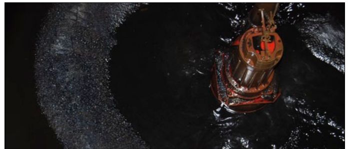
Inside the lift station: A Bravo 40 slurry pump
