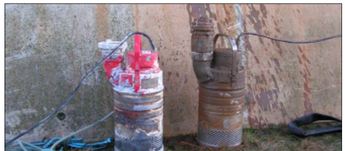
After 3 months, the aluminum pump (left) have corroded heavily, while the INOX pump (right) is doing just fine.
