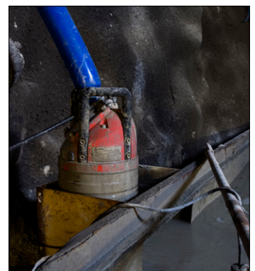
A Major pump in another sedimentation tank
